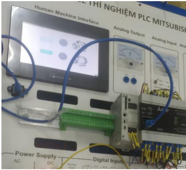
Figure 4: HMI connected to the PLC via Ethernet, enabling real-time control and monitoring of system processes
